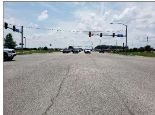
Figure 14: Deteriorating Pavement in 9th Street Corridor
