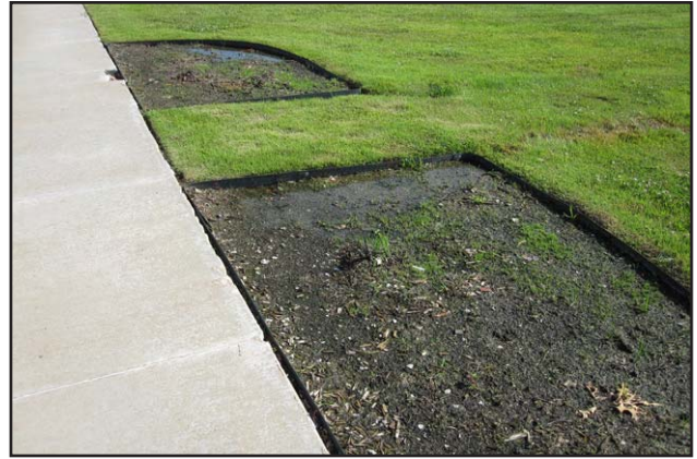
098 - East side drainage issue adjacent to sidewalk on 100 Block of S Main St
