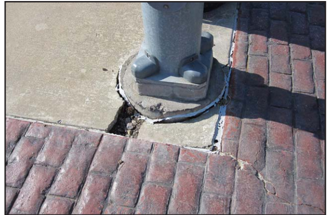
100 - East side brick pavement and stop light footing at Southeast corner of S Main St & E Broadway Ave
