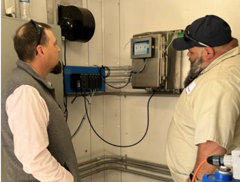
Engineering & Construction Department Director Ethan Edwards and the Environmental Division attended a NEXICON Multismart Information Training held by Utilities Department at the Berwick Lift Station.
