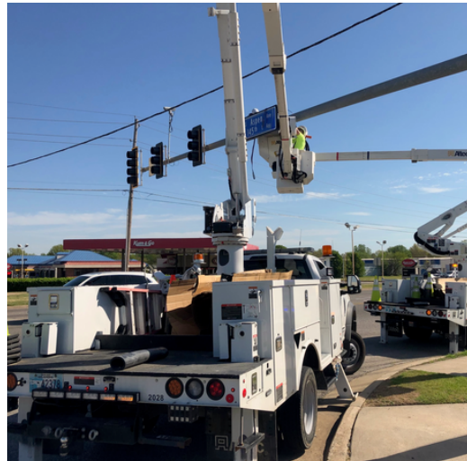
City crews install new LED Street Name Signs at the intersection of New Orleans St. and Aspen Ave.
