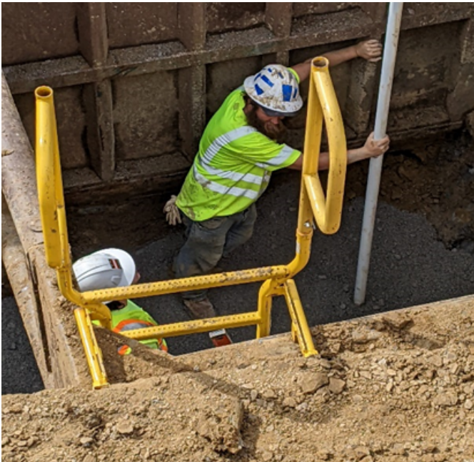
David Lloyd checks the grade for a sewer main line on 37th Street.
