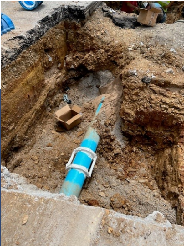
Utilities crews installed an insertion valve near St. John Hospital in north Broken Arrow.
