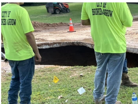
City crews inspecting a sinkhole.
