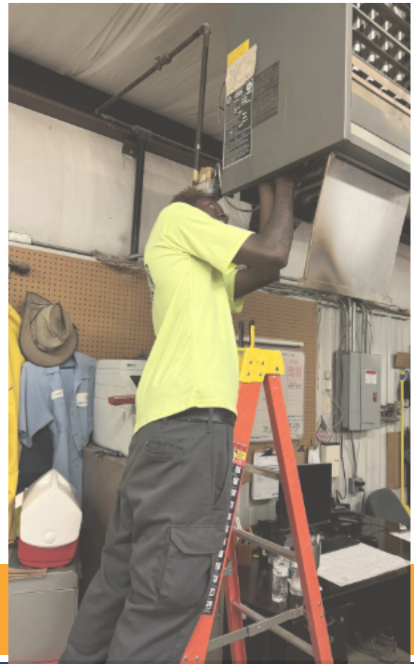
TJ Mayfield, who has recently started working for the City of Broken Arrow, is already finding himself right at home as he works on a heater that services the shop area at Park Grove Cemetery.
