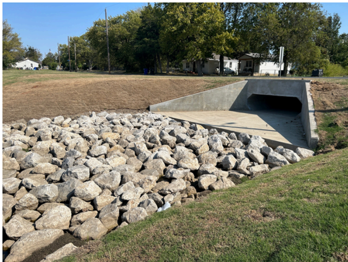
A view of the Elm Avenue Culvert Replacement Project just east of Elm Place between Kenosha and Houston streets.
