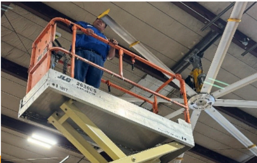
Moku Funk is currently working on the large fans at the Fleet facility. He began his career with the Building Maintenance Department in October of 2012, and this month marks 12 years of dedicated service.
