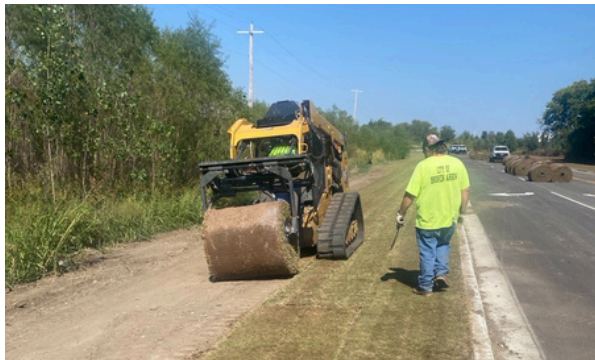
Stormwater crews laid more than 160 rolls of sod on the new 43rd Street. With a little more work, the first phase of this new road will be complete.
