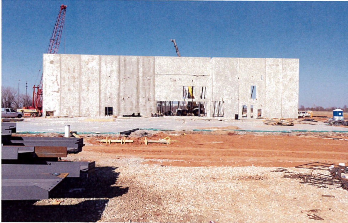
Photo 1 – The South wall of the Core (Grands & Lobby) area. By week's end this area will be enclosed on three sides (back and two sides). Walls on the north stadium wing could start next week (they are setting forms and pouring walls now).
