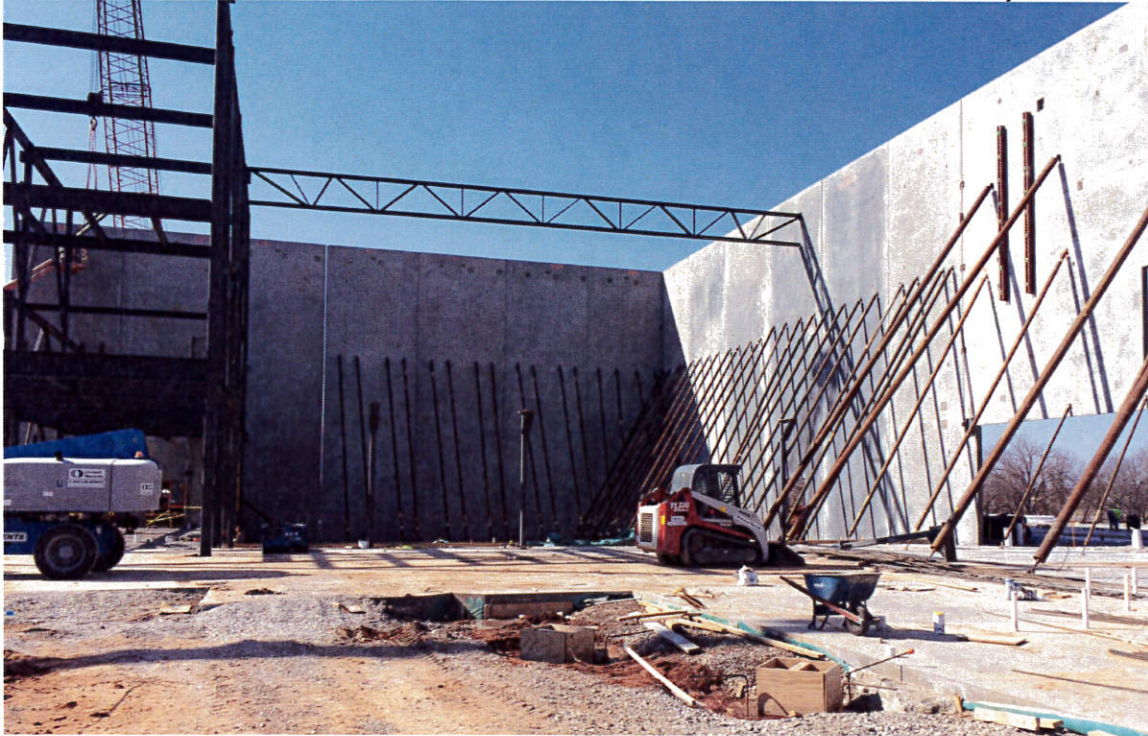
Photo 3 – Closer look showing the roof truss. They are prepping for more roof work.
