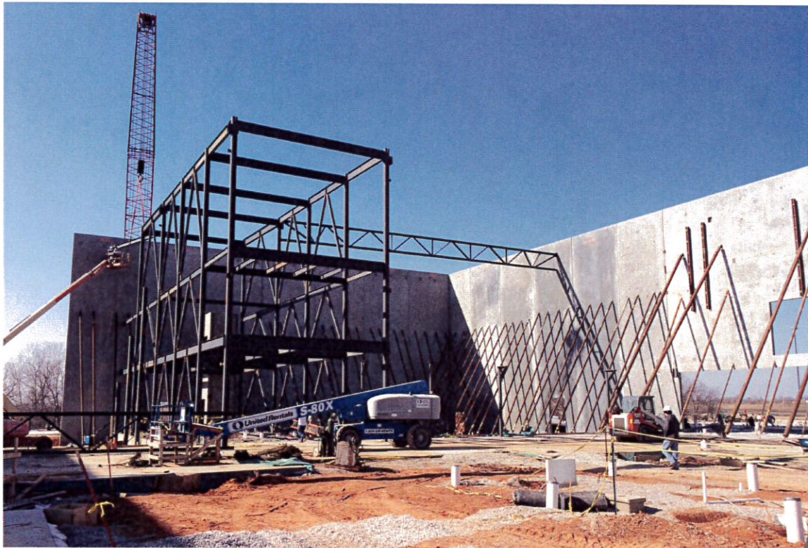
Photo 2 – Steel is moving along well and there is a lot of steel on site so work will not be impeded by lack of material. Note the FIRST roof truss spanning #8 Grand.
