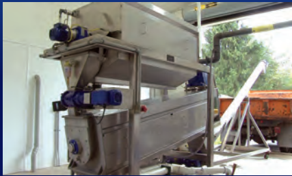
DSP Screw Press Model 3012, NY WWTP
