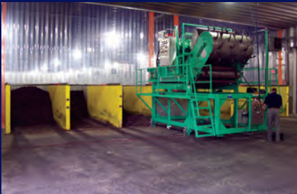
Agitated and Aerated In-vessel type Composting System (ICS)
