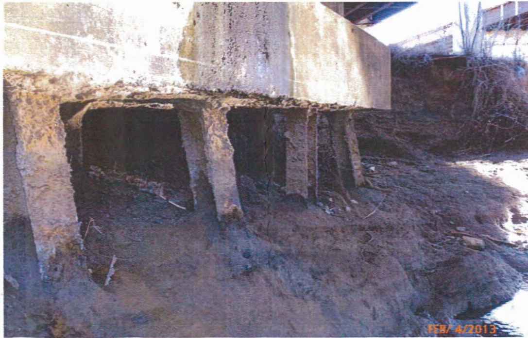
Exposed piles at East abutment
